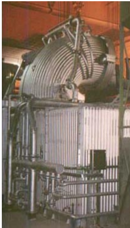
FOURTH HOLE Settling chamber on an Electric Arc Furnace Application
