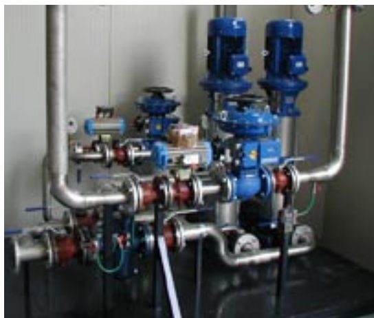
SPRAY SYSTEM VALVE RACK For precise temperature regulation
