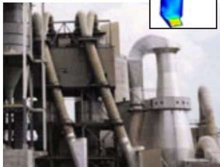
COOLING TOWER for cement preheater kiln
