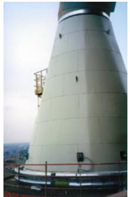
SPRAY LANCE HEADERS Water and compressed air distribution to the lances
